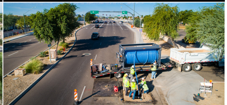
Arrowhead Ranch Water Reclamation Facility WAS Line Rehabilitation / CMAR / City of Glendale
